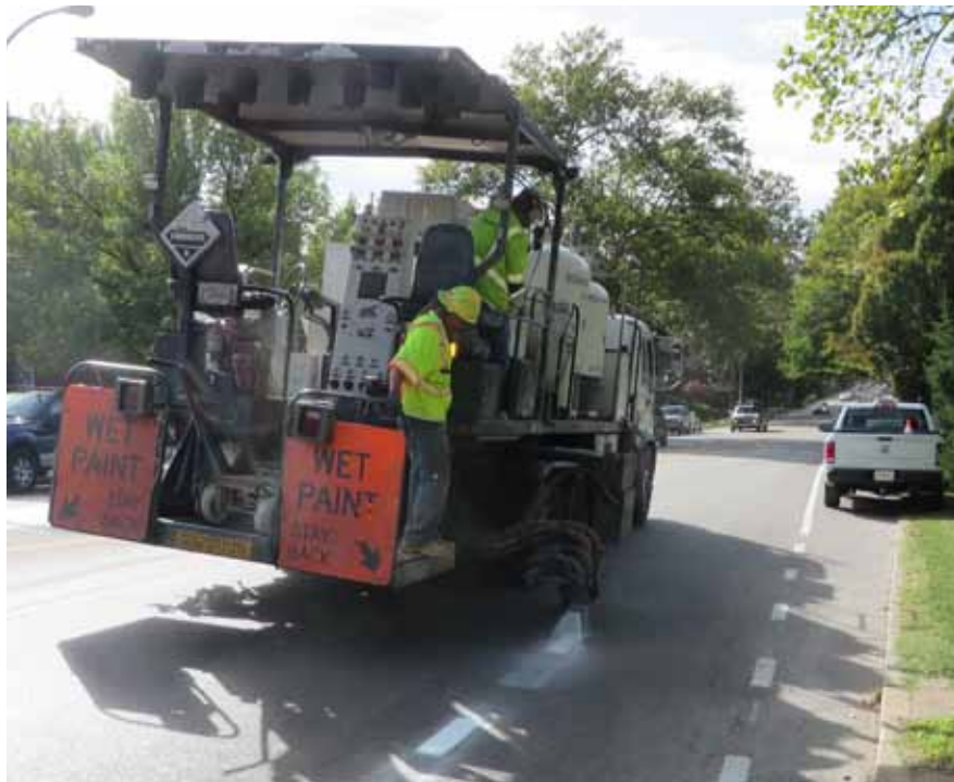
Figure 6.23: Lane restriping is an essential component of any bike lane or cycle track project.
