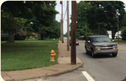
Figure 2.16: The lack of a curb ramp and narrow functional width of the sidewalk make this a difficult environment for users with mobility impairments, or even two pedestrians walking side by side or passing each other (location: Weinbach Ave)
